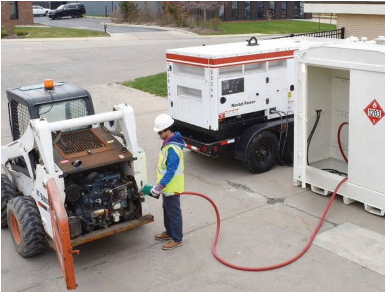
Fuel Island is a self-contained, moveable fuel station that can be deployed for fleet refueling as well as long-term, stationary applications. CREDIT: WESTERN GLOBAL
