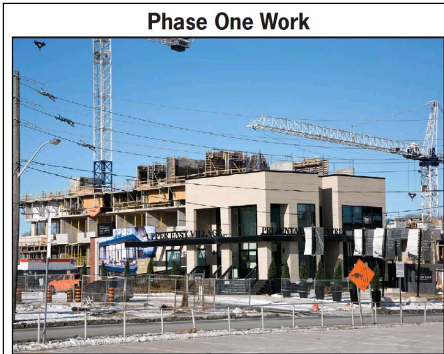
Construction is progressing for the Upper East Village mixed-use development phase one on Eglinton Avenue East in Toronto. The developers are Camrost-Felcorp/Diamond Corp. and the work includes one 21-storey, 283-suite tower and one 18-storey tower with 231 suites and three levels of underground parking. The amenities will include a fitness/yoga centre, indoor pool, party room, rooftop terrace with barbecues, a half-acre park with outdoor gardens and a fire pit lounge. The project was designed by IBI Group and consultants are Odan Detech Group Inc. (civil), Powell & Bonnell (interior) and Janet Rosenberg (landscape).
